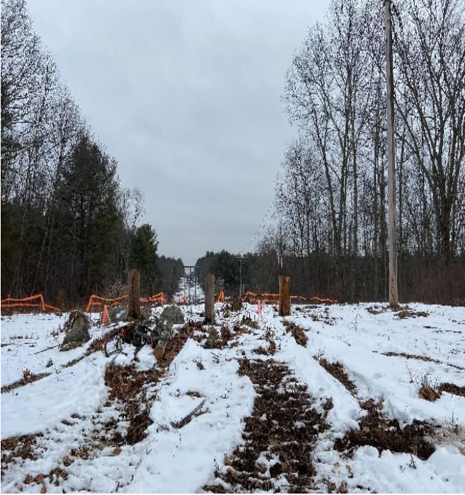
Fig 5: Existing poles removed in the location where Str. 58 is to be drilled. Viewing east. (12-27-19).
