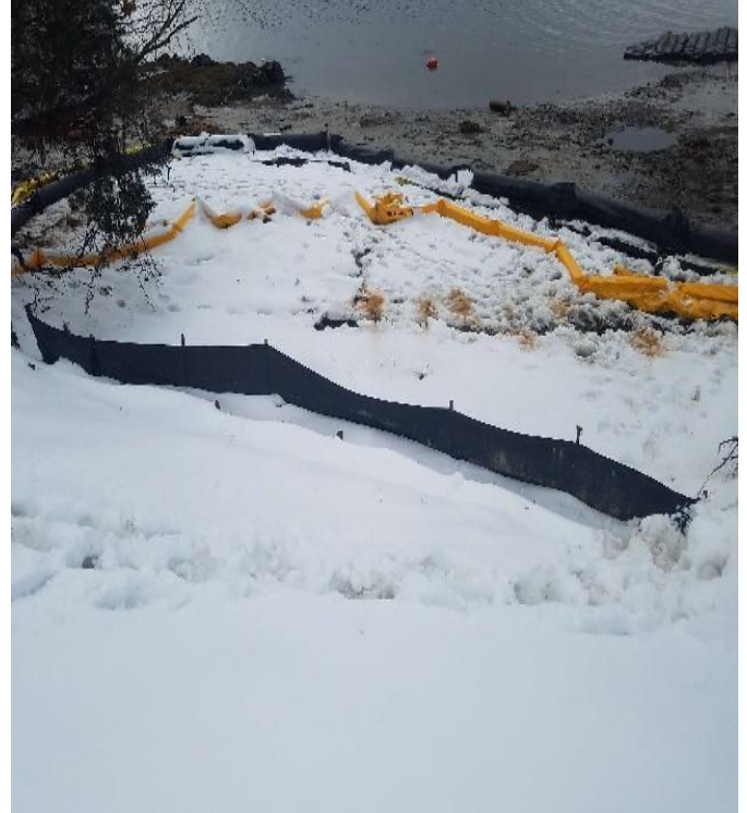
Fig 14: Sediment controls functioning well at Gundalow Landing/east side of the Bay. Viewing southwest. (12-31-19).
