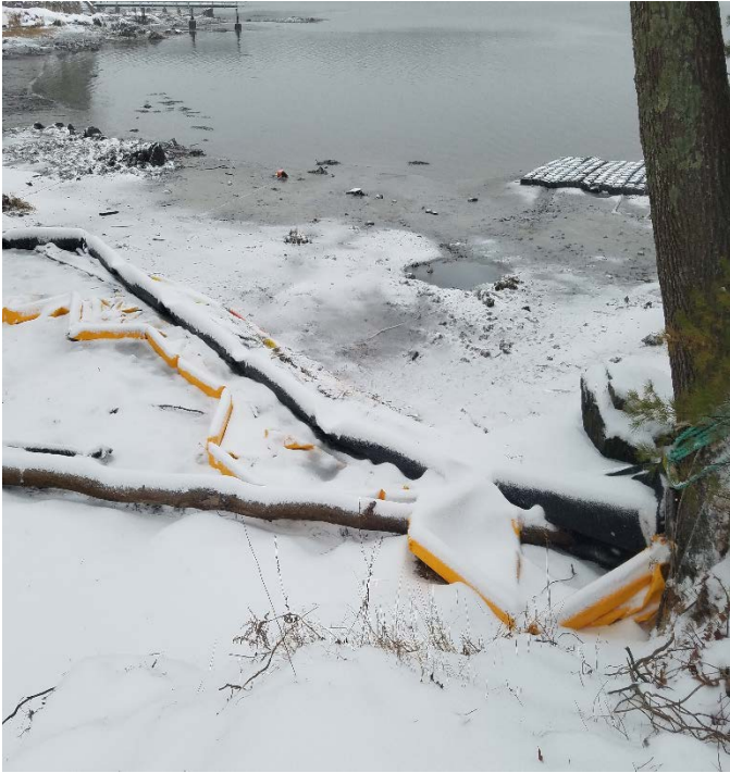
Fig 9: Turbidity barrier installed in intertidal zone at Gundalow landing/ East side of the Bay. Viewing east. (12-30-19).
