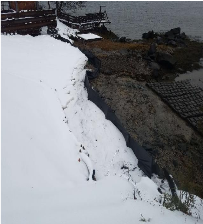
Fig 11: Sediment controls functioning well at Getchell property/west side of the Bay. Viewing south. (12-31-19).
